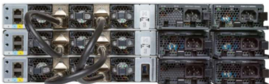
Figure 5. Cisco Catalyst 9300 Series switch stack units
