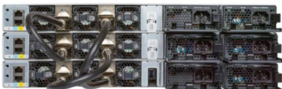
Figure 5. Cisco Catalyst 9300 Series switch stack units
